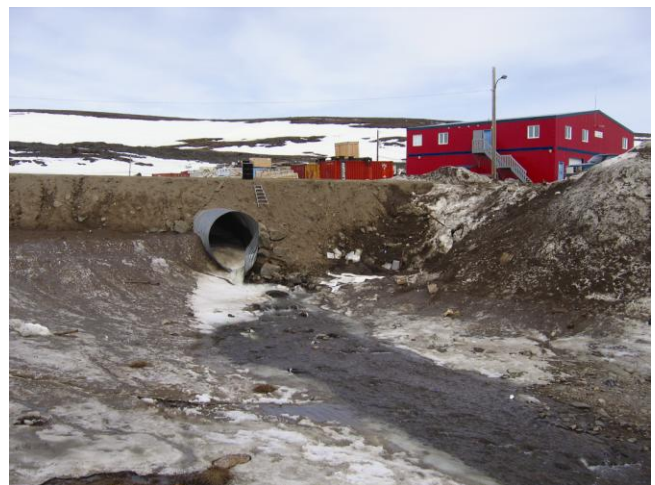
Oil runoff through road culvert.
