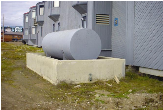
1,000 gallon oil tank in concrete berm.
