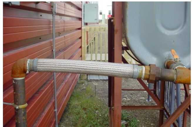
Stable fuel tank on a metal stand with flexible connector.
