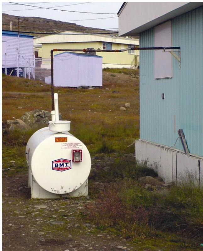
Oil tank with unsupported fuel line.
